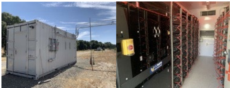
Figure 3: 300 kWh repurposed storage system at the UC Davis Robert Mondavi Institute Winery (Photo credit: M. Slattery)
