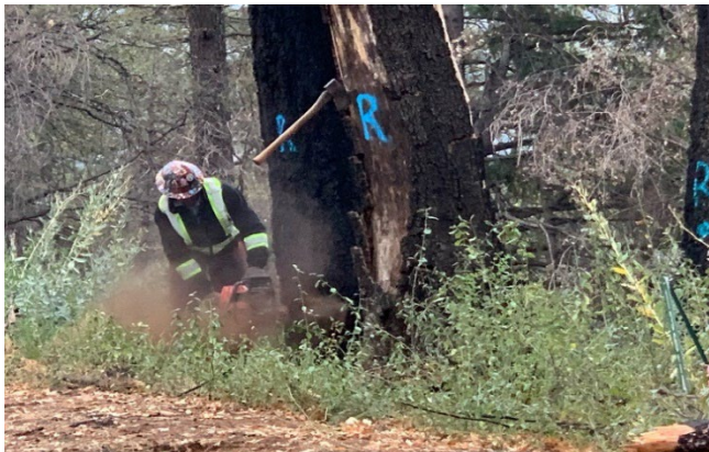
CalRecycle contractors removing hazard trees in the Camp Fire burn scar. Photographer unknown.
