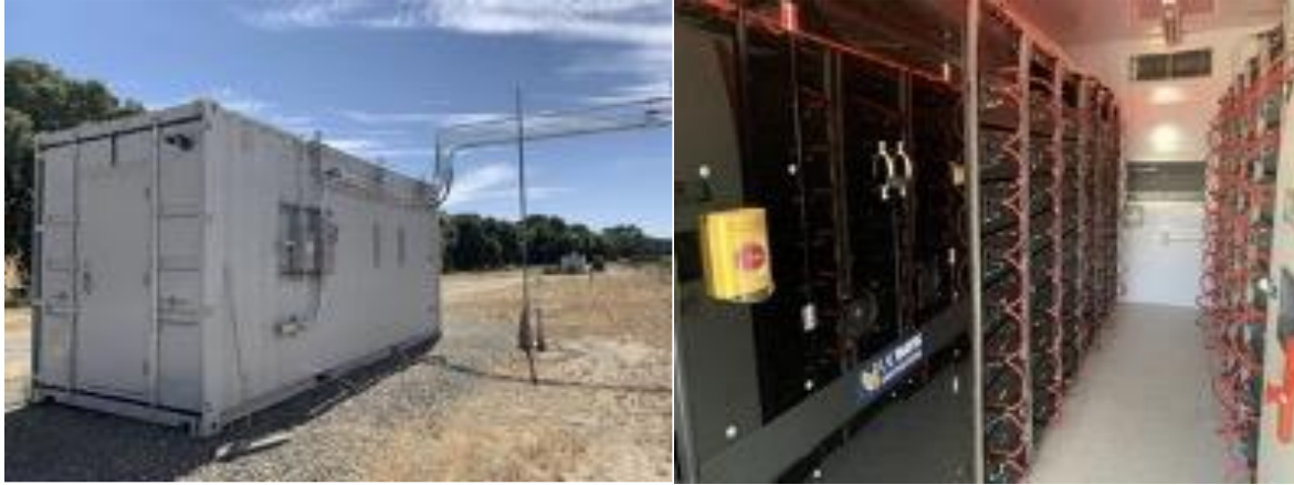
Figure 2: RePurpose Energy's 300 kWh system at the University of California, Davis Robert Mondavi Institute Winery (Photo credit: M. Slattery)
