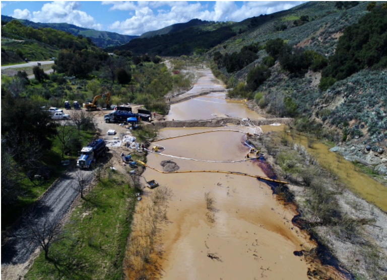
Aerial view of emergency cleanup activities, including temporary dams provided by Central Coast Regional Board staff. Photographer unknown.
