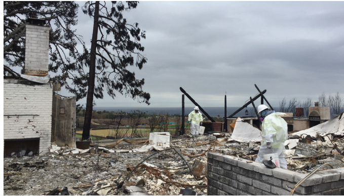
DTSC HazMat crews assessing a residential structure destroyed by the Woolsey Fire in Los Angeles County.
