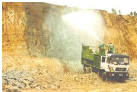
A truck applies chemical stabilizers to reduce soil erosion where vegetation can not be planted (Source: Terra Firma Industries, 1999)
