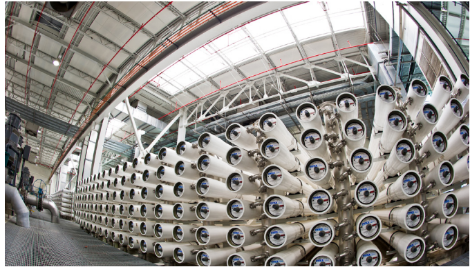
County Water District uses reverse osmosis to treat wastewater for its seawater intrusion barrier.
