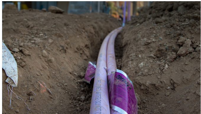
Pipes, laid in 2015, carry recycled water to irrigate residential property in gated Serrano subdivision in El Dorado Hills.
