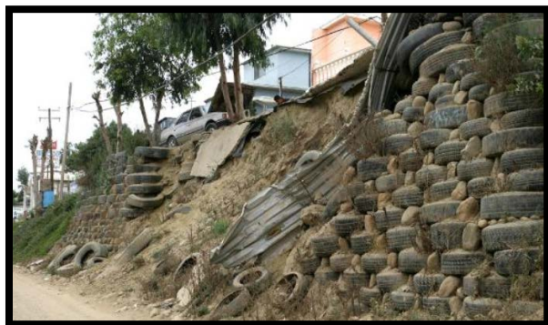
Figure 9 Failed retaining wall, which threatens the integrity of the upper road and the lower road. Tires often end up in the canyon bottom and are transported downstream into the United States. Source: 2009 Waste Tire Study
