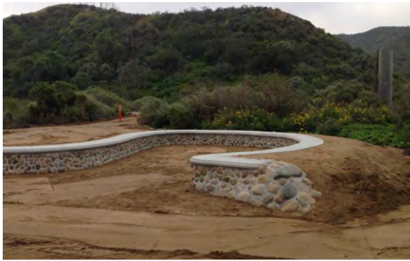
Border Gateway to Nature project to build a seat/wall complete. Image Courtesy: Chris Peregrin, California Department of Parks and Recreation
