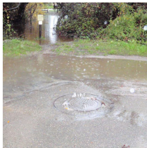
Sanitary sewer overflow in San Luis Obispo
