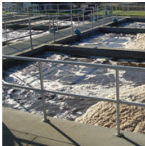
Typical activated sludge basin at a wastewater treatment plant.
