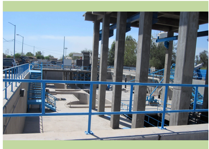
Trash screen and pumping station in Mexicali.
