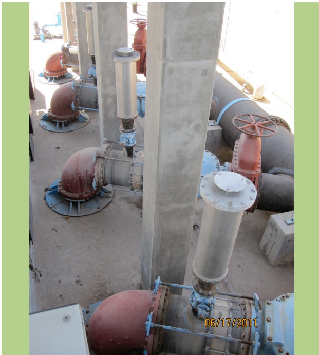
Pump Station in Mexicali
